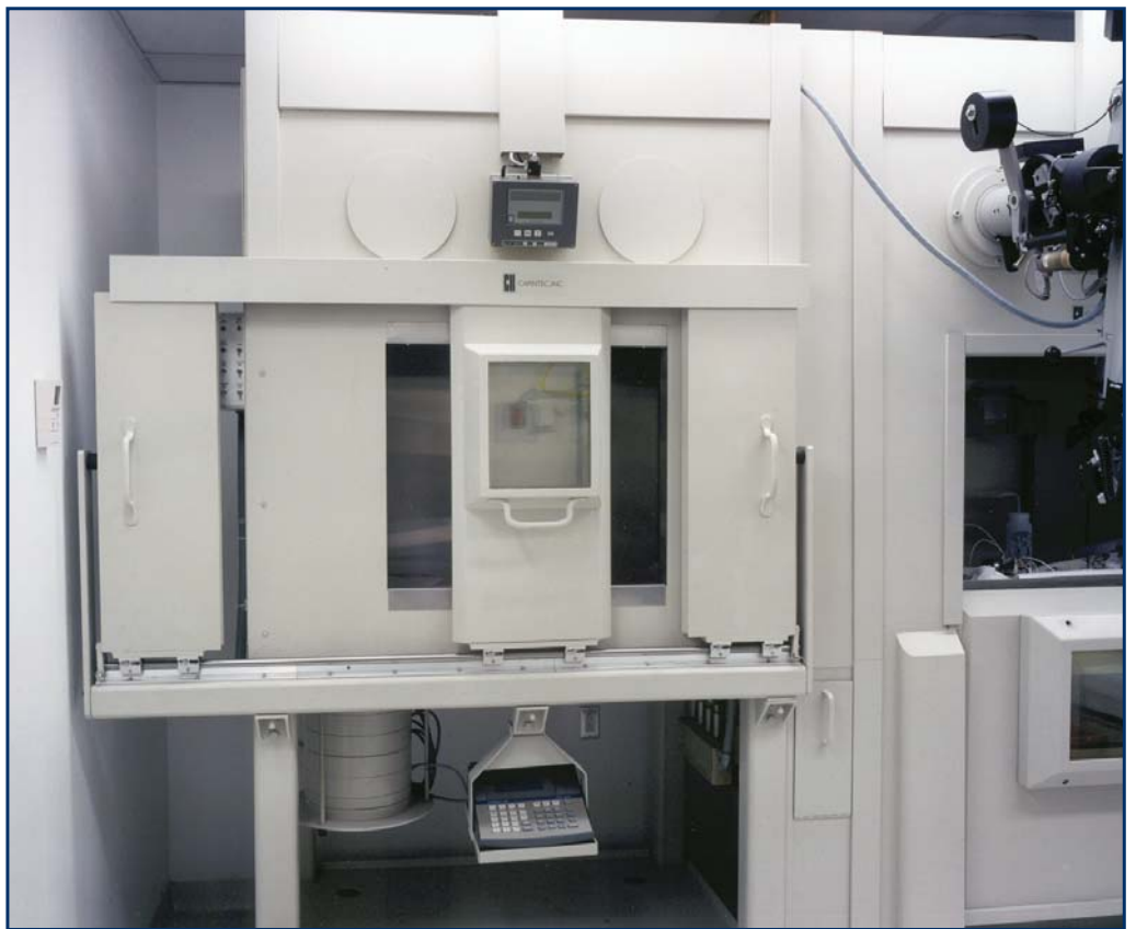
Hot cell with 3 piece horizontal door design shown with body shield in place for effective radiation protection
